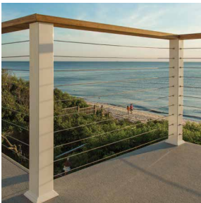
Horizontal Cable shown with wood posts and vinyl sleeves
